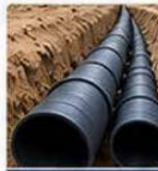
STORM WATER DRAINAGE
