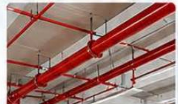
FIRE PROTECTION PIPING
