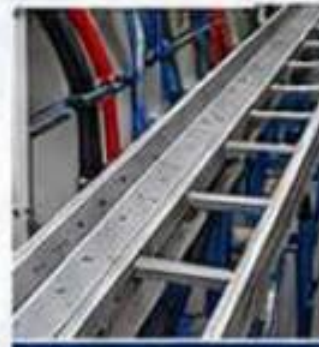
CABLE TRAY & TRUNKING
