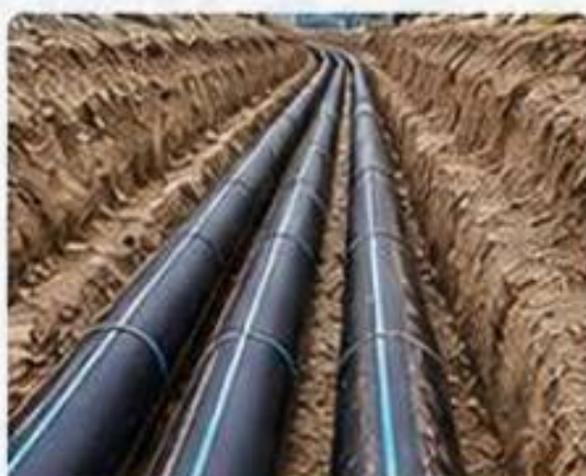
UNDERGROUND HDPE NETWORKS
