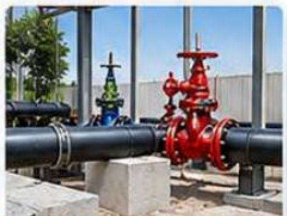
HDPE FIRE PROTECTION NETWORKS
