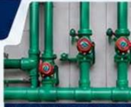
DOMESTIC WATER SUPPLY
