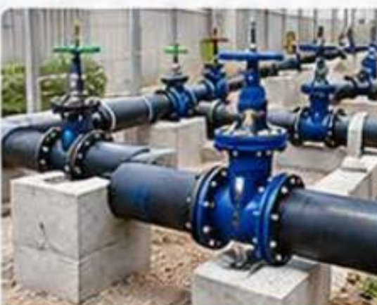
HDPE WATER LINES
