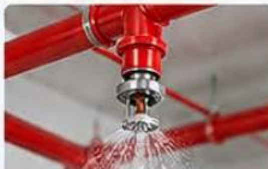
FIRE SPRINKLER SYSTEMS
